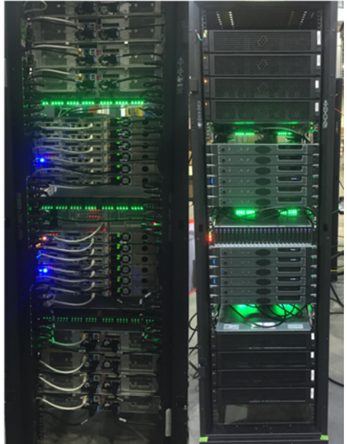
Fig. 1. COMPaaS Hardware Racks
