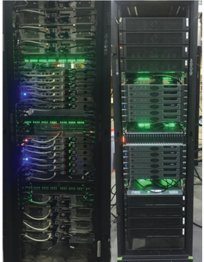
Fig. 1. COMPaaS Hardware Racks
